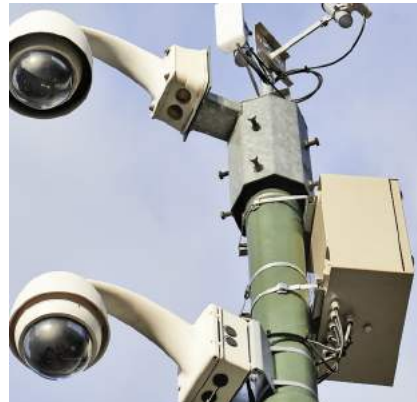
Surveillance and CCTV Systems
