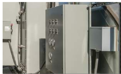
Rooftop Control Systems
